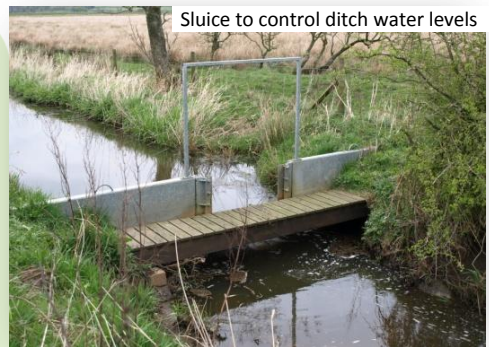
Sluice to control ditch water levels
